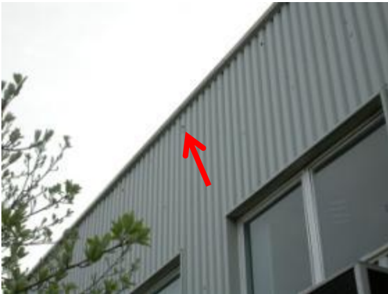
Fig. 9 Metal cladding with hole (arrowed)
